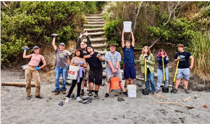
Volunteers with Upward Bound TRIO making repairs to the Baker Beach trail cable steps.
