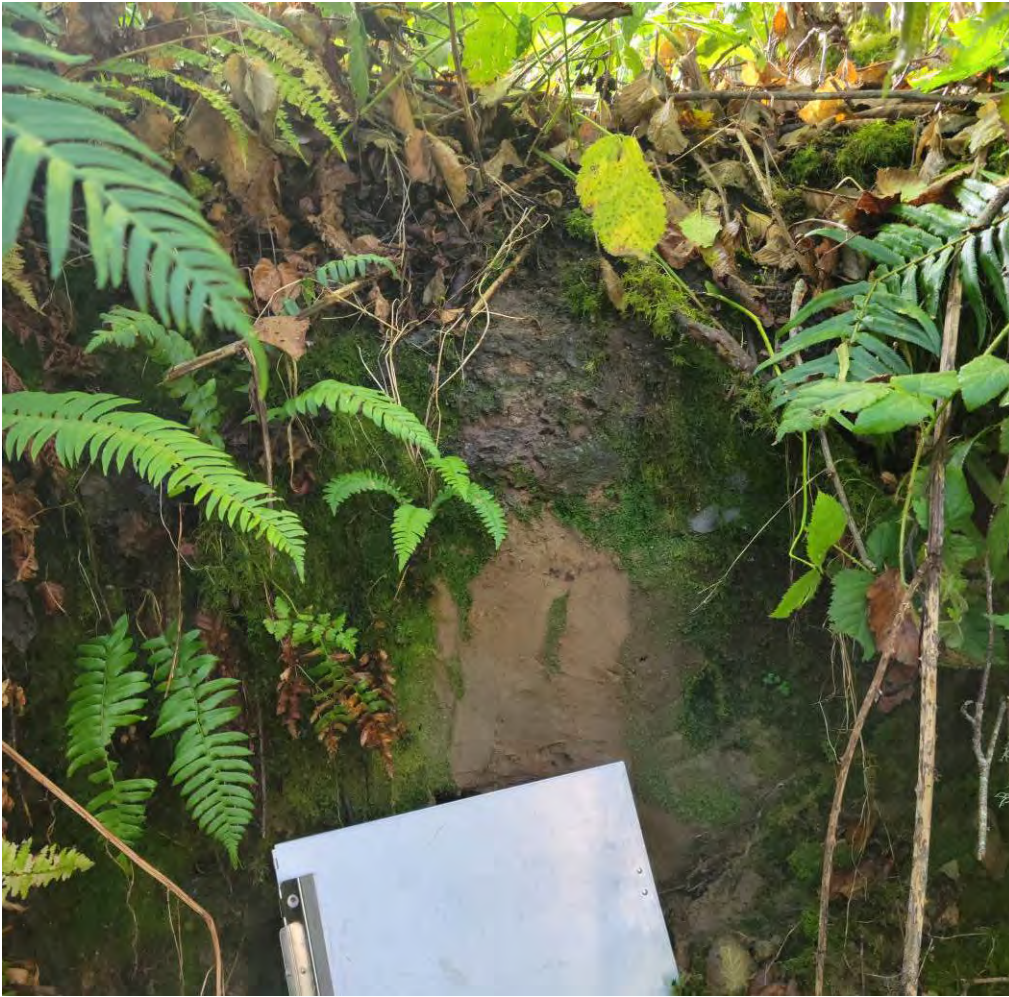
Photograph Location No. 8, Photo B: An exposed section of buried road base resting on sand, immediately downslope of the corrugated metal culvert.
